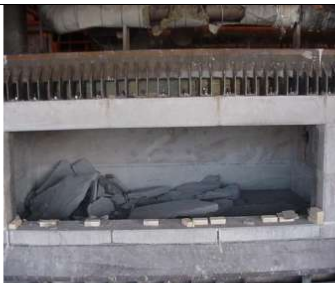
Figure 14: Explosive spall in the hearth of an aluminum melting furnace.
