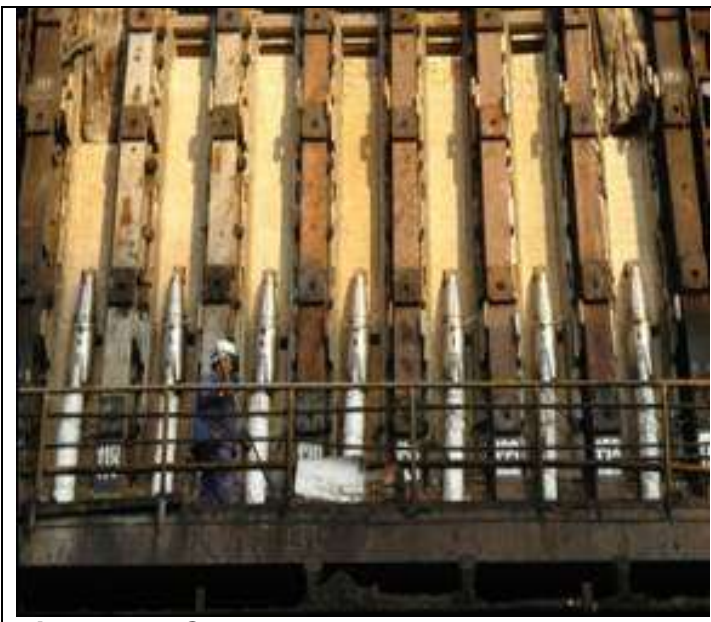
Figure 22: Conventional slot oven coke battery
