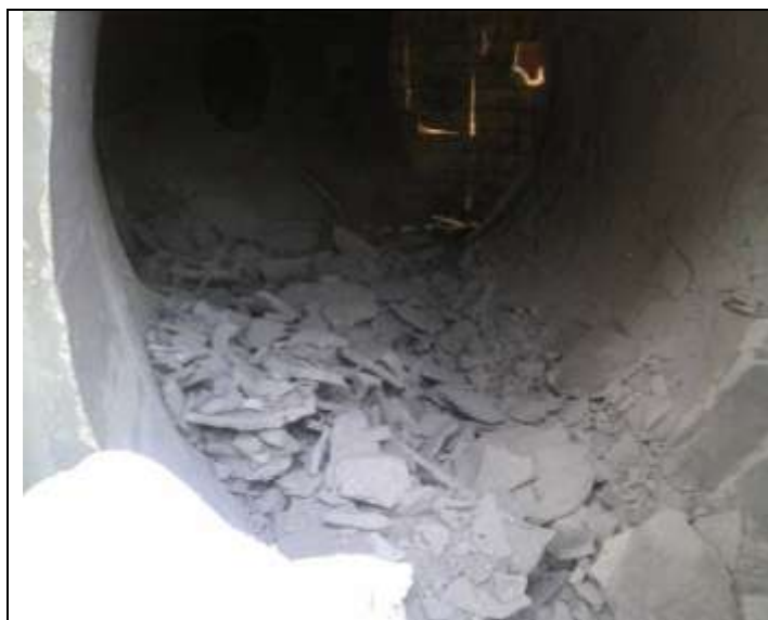
Figure 13: Explosive spall in a refractory lined duct.
