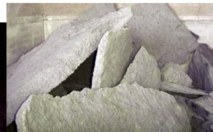
Explosive damage occurs when high pressure steam can not escape, often at 425° C.
