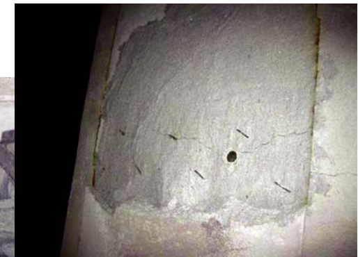
Steam pressure damage.
