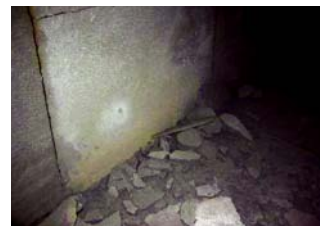
Damage from localized radiant heat. Breakage is thinner and of a smaller size.
